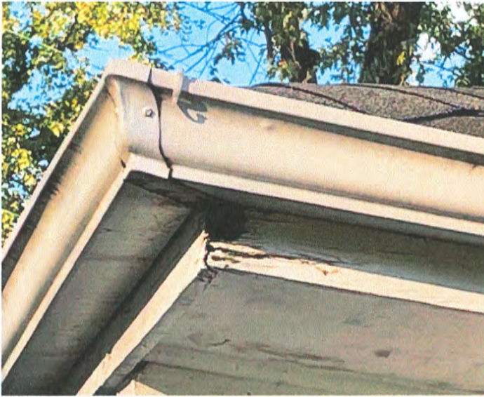
886 Dewberry Ct - Gutter/eaves damage SW corner
