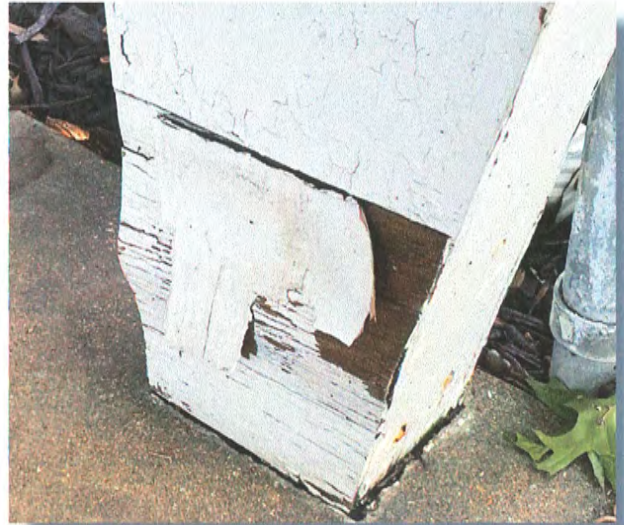
Pillar damage SW corner
